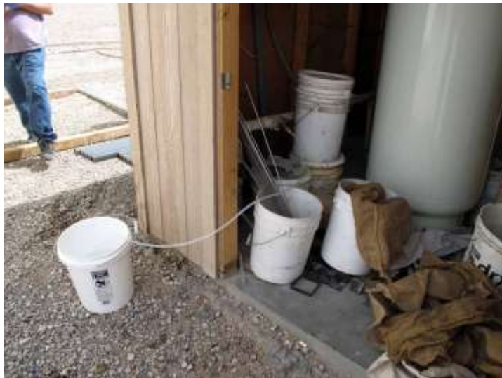
Bypassing pressure tank to collect sample from non-flowing domestic well after completion of purging.
